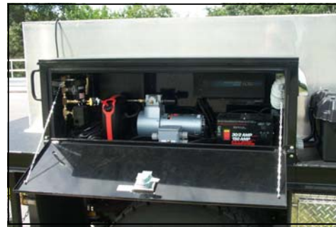
Equipment Housed in Weatherproof, Lockage Enclosure
